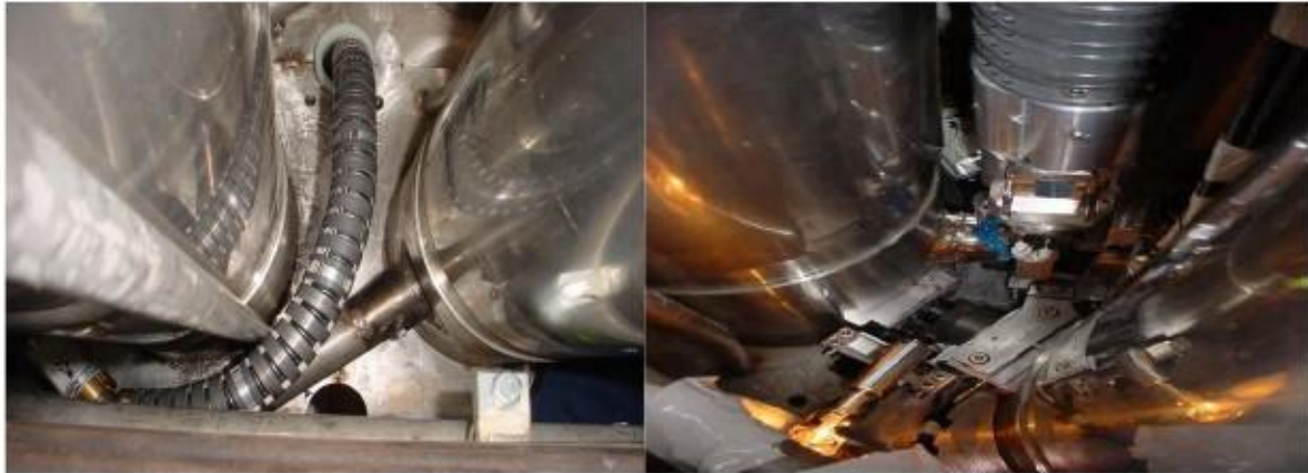
Ringhals Inspection Arm
