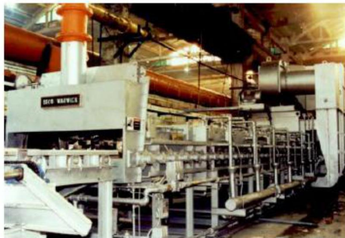
Figure 2.3 Fuel Fired Furnace
