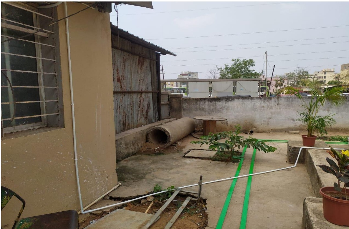
Waste Water Treatment Plant
