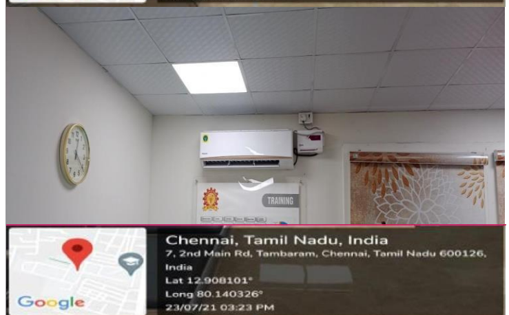
Wi-Fi Sensor based automatic lighting system installed in the BIHER campuses
