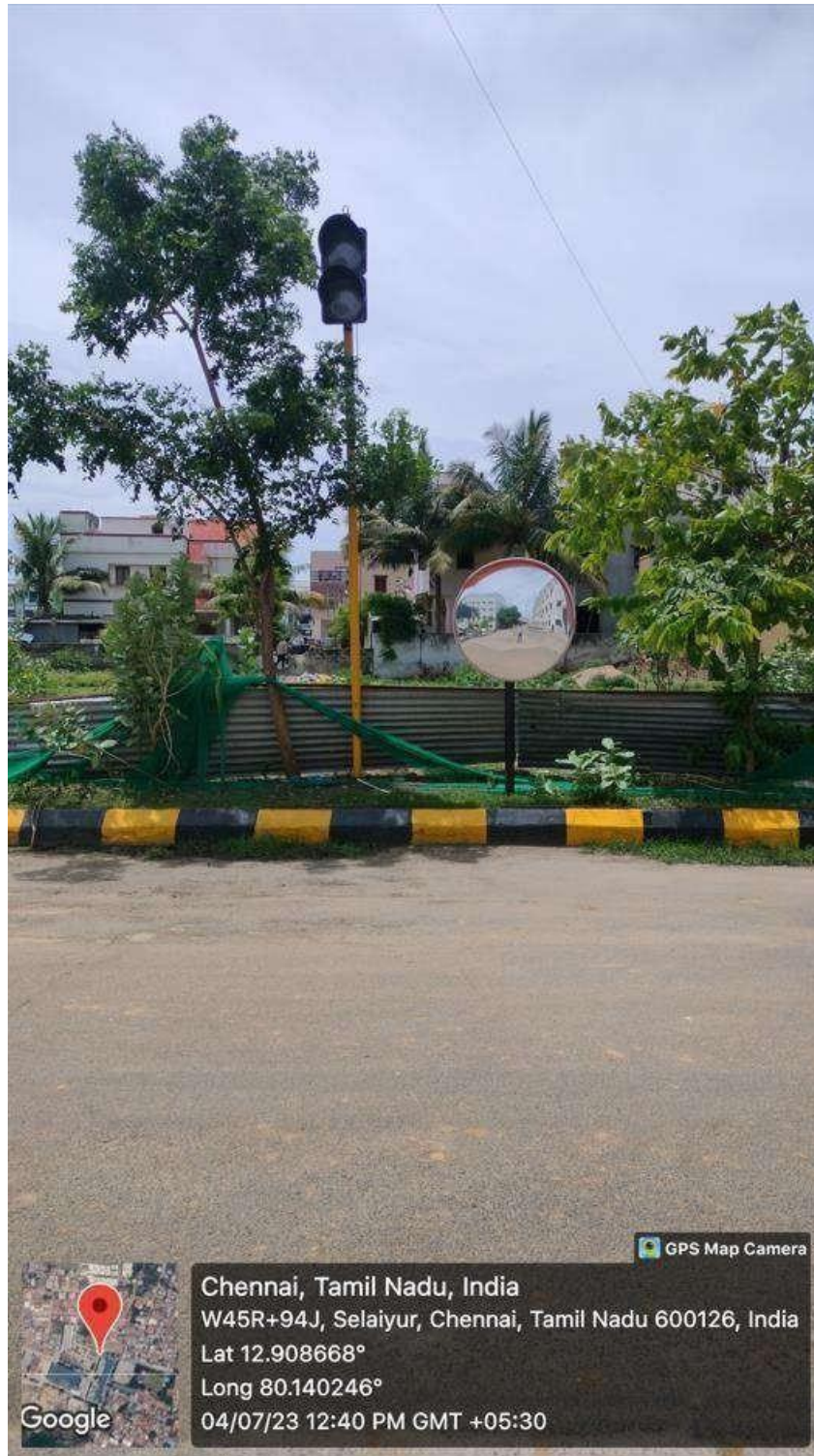
LED Traffic Lights inside the campus
