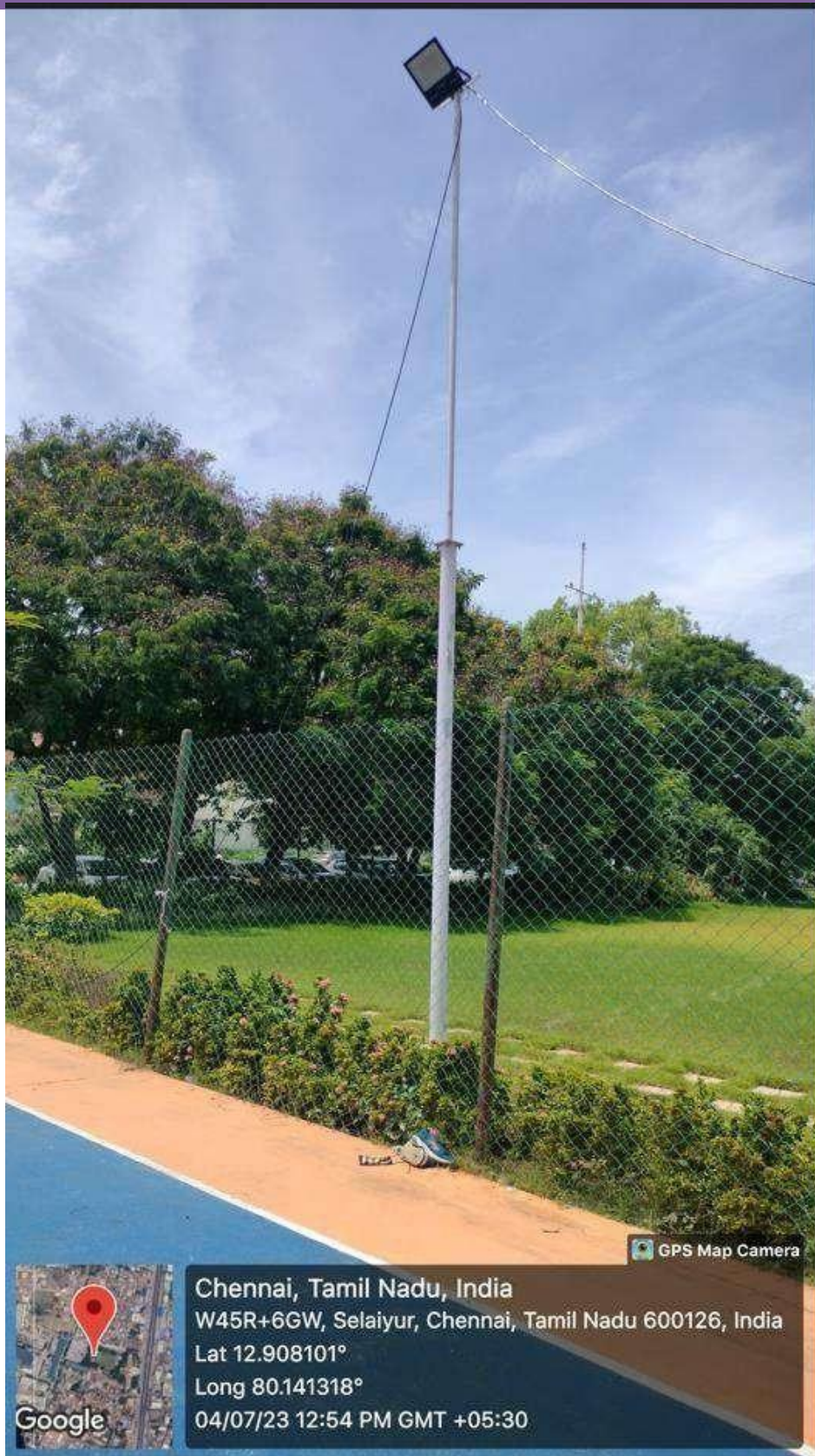
LED Street Lights inside the campus
