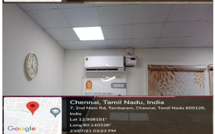
Wi-Fi Sensor based automatic lighting system installed in the BIHER campuses
