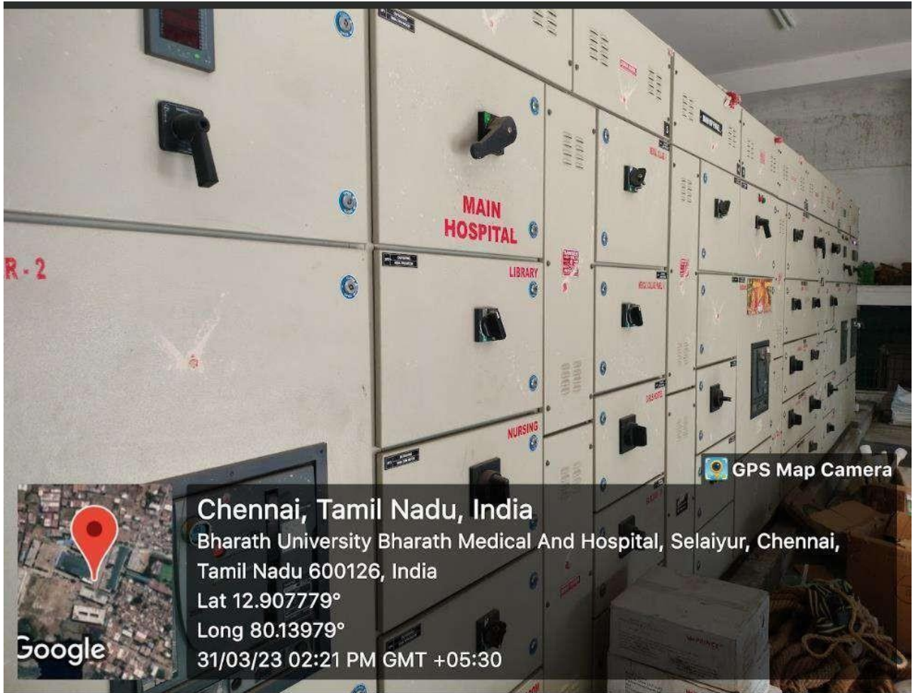
Electrical Panel Room
